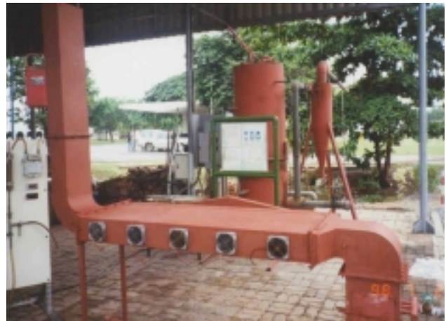
Figure 2: Biomass stove-heat exchanger unit, before insulation
