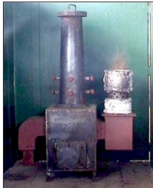
Figure 3: IGS-2 in operation
